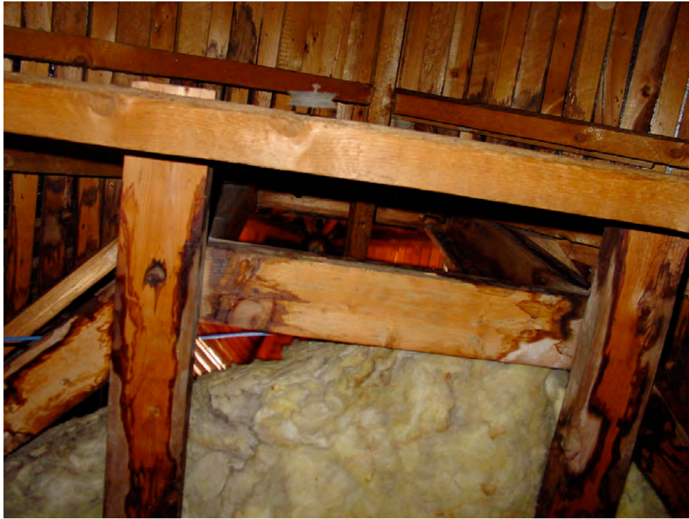
EC-2a: Looking up into cupola from roof void. Note water stains.
