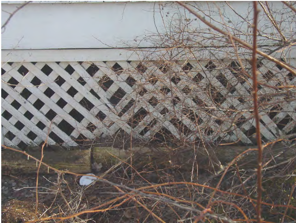
EC-7: Deteriorated trellis.
