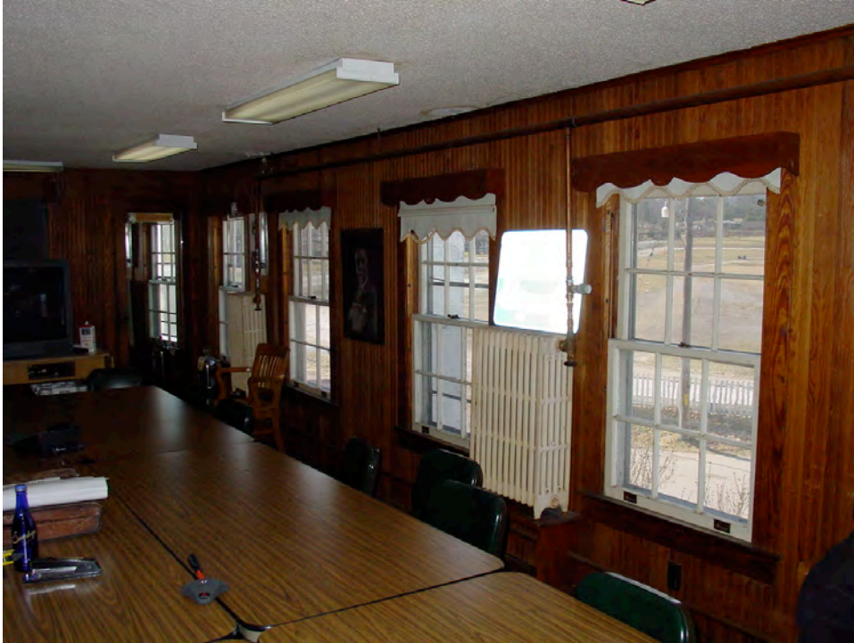
IC-5c: Radiators in current second floor meeting room, again, elevated to operate as a two-pipe system.
