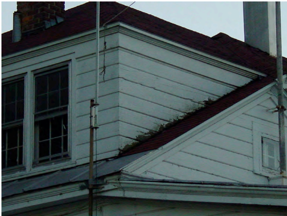
EC-2b: Dormer flashing which leaks, east end of main roof.
