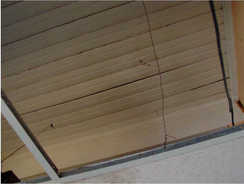
IC-2c: Water damage to bead board ceiling.
