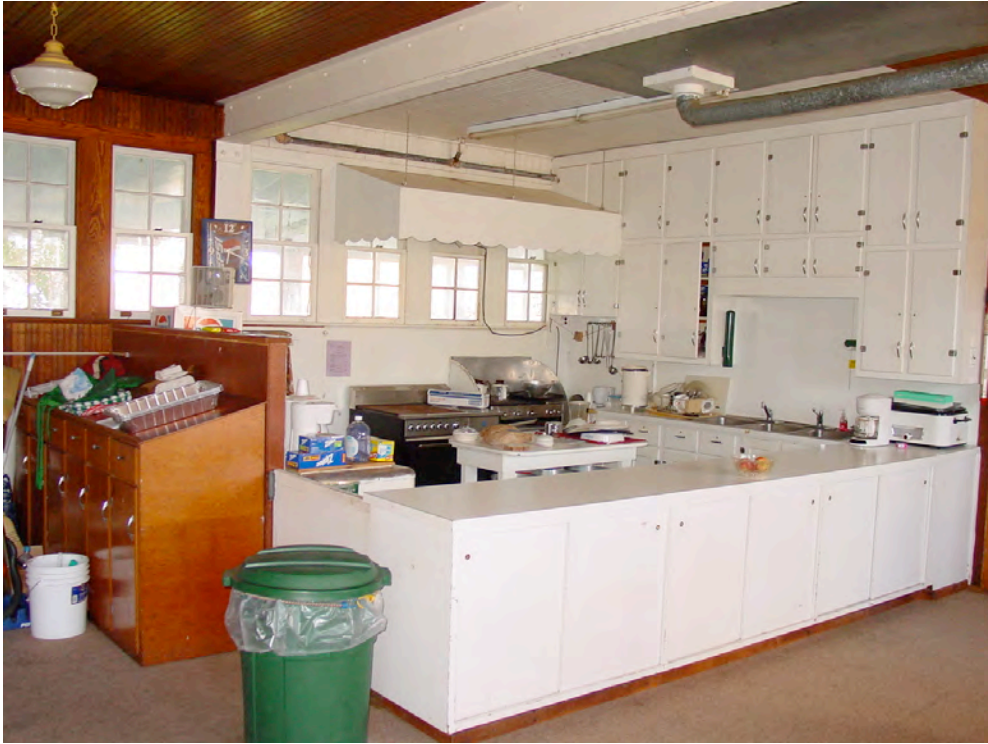
PR-4: The kitchen, as is, with no separation from the main space.
