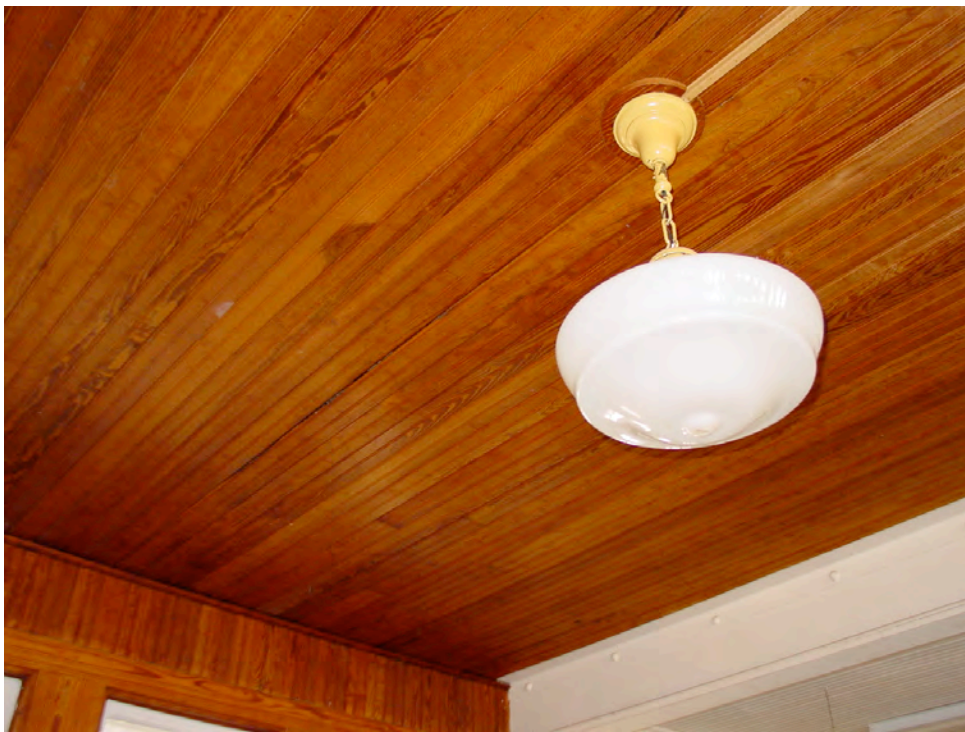
IC-3b: Schoolhouse light fixture in main assembly space.
