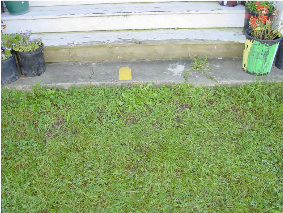
EC-4c: Broken concrete stoop at north portico.
