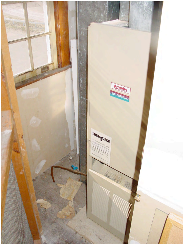
IC-5d: Furnace on second floor, west.
