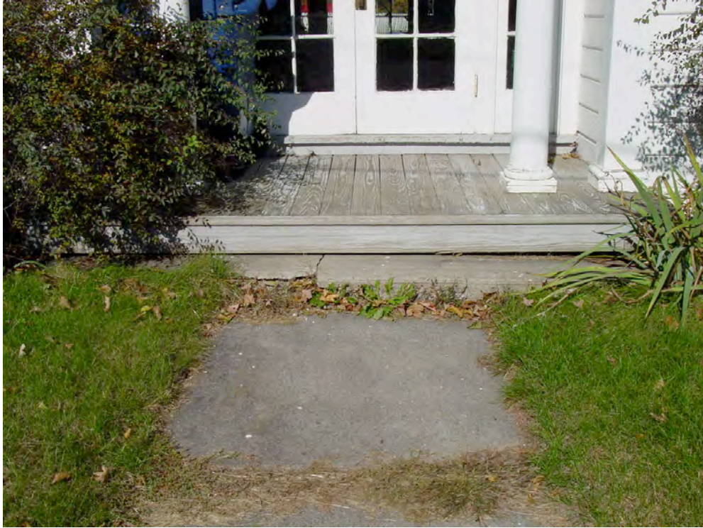
EC-4b: Broken concrete stoop at south portico.
