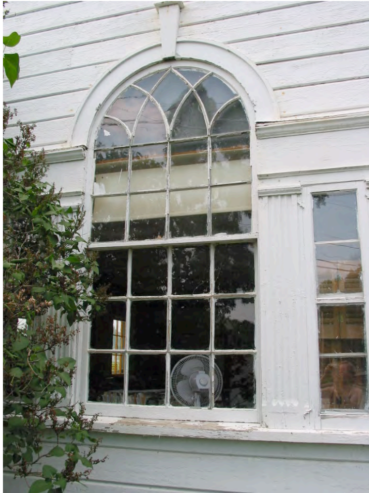
EC-3a: Palladian window in need of repair and maintenance. Note missing plinth on pilaster.
