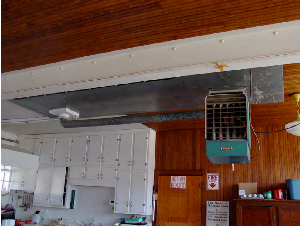
IC-5e: One of two propane heaters in main assembly space. Note metal shield over flue pipe on ceiling.
