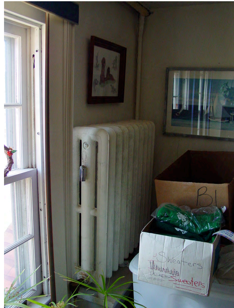
IC-5b: Typical steam radiator, elevated to improve condensate return.
