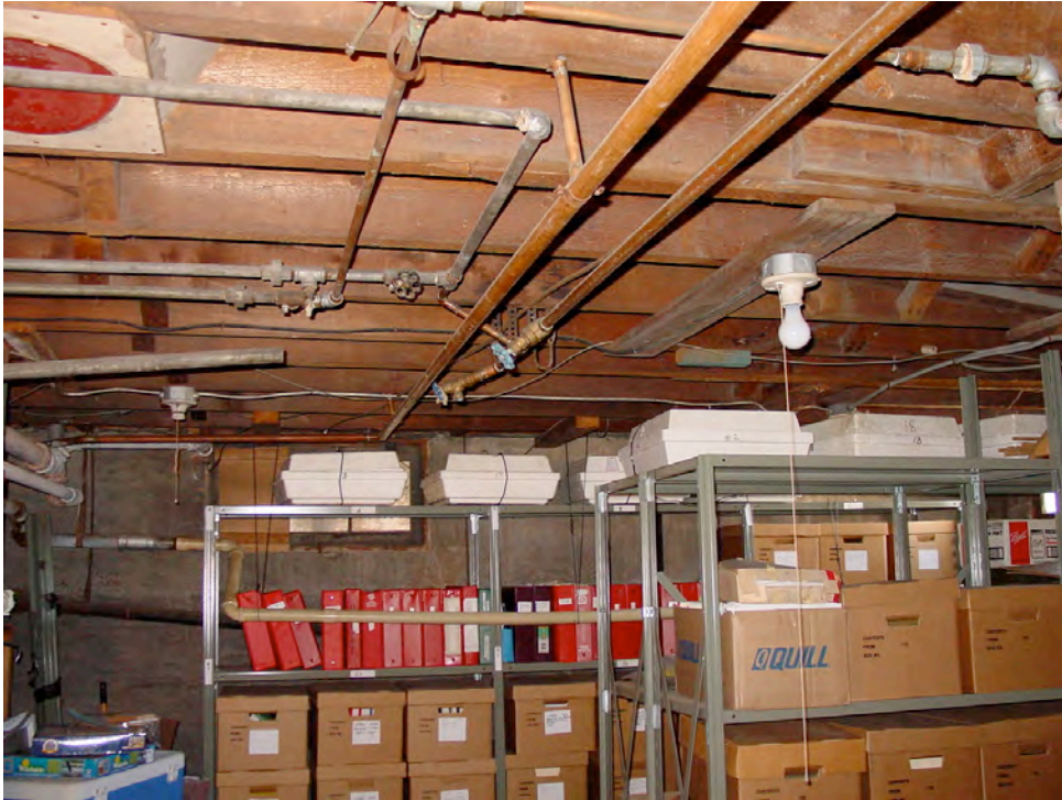
IC-4a: Basement plumbing, a mixture of threaded iron and soldered copper.
