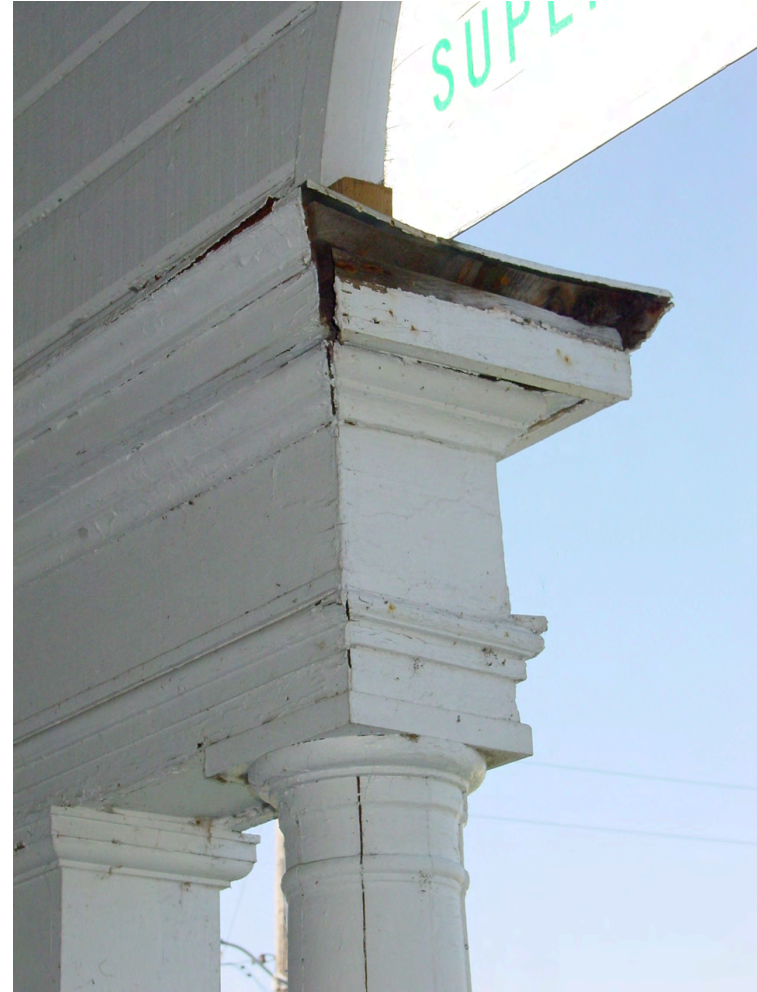
EC-3b: Detail of entablature at north portico missing crown and portion of tenia molding.
