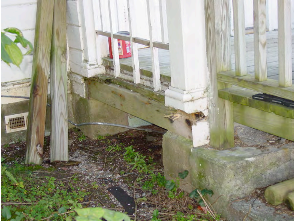
EC-5a: Porch edge rotted away at northwest entry.
