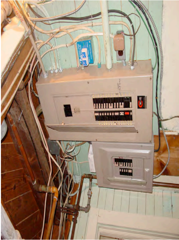
IC-3a: Electric panel in basement.
