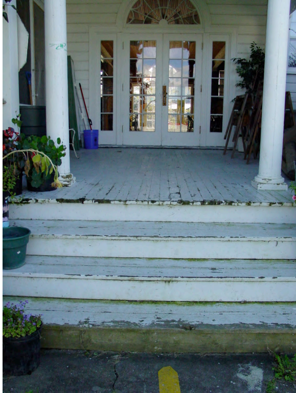
EC-5c: Decking starting to weather at north portico
