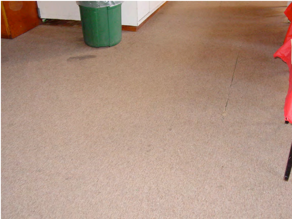
IC-2d: Stains and tear in carpet in main assembly space.
