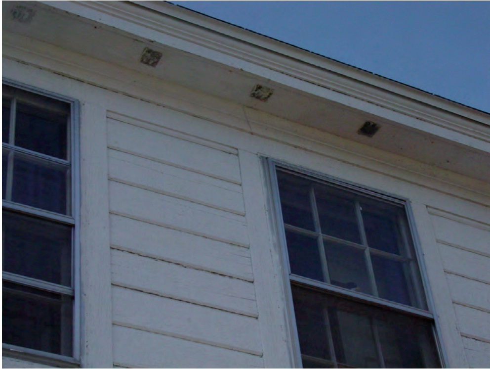
EC-6: Rusty vents in planceer piece (soffit).
