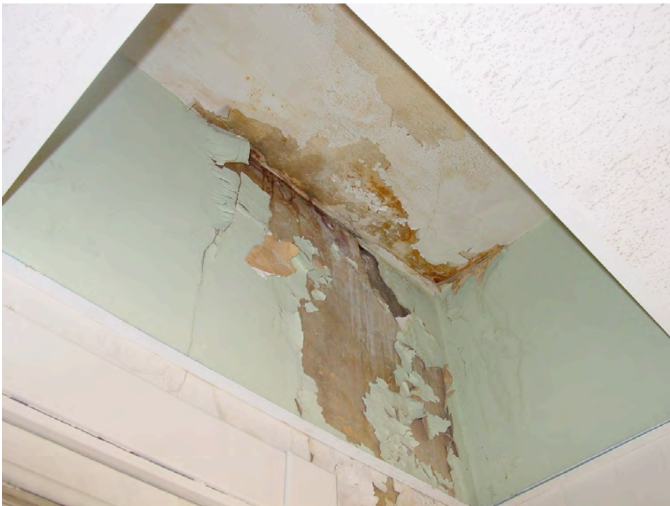
IC-2b: Water damage to plaster and paint finishes.
