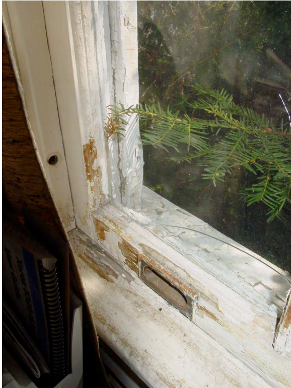
IC-2a: Detail of paint deterioration on window components.
