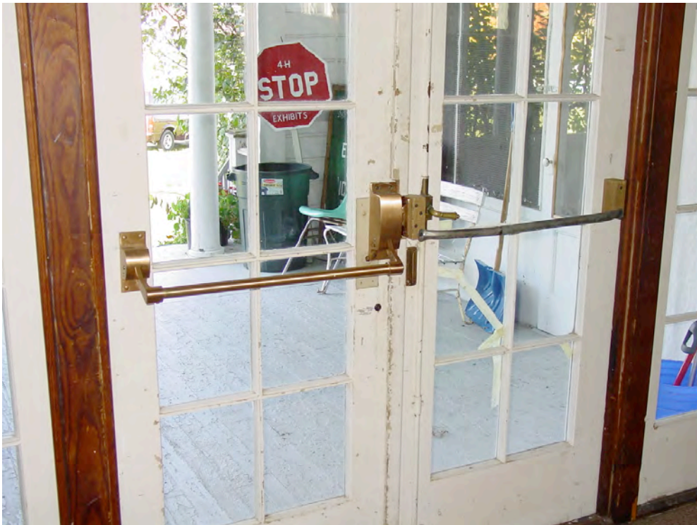
PR-1b: Assembly space, homemade hardware on inactive leaf of exit door.
