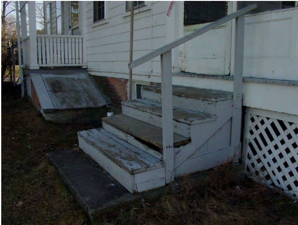
EC-5d: Deterioration at east steps to north porch.
