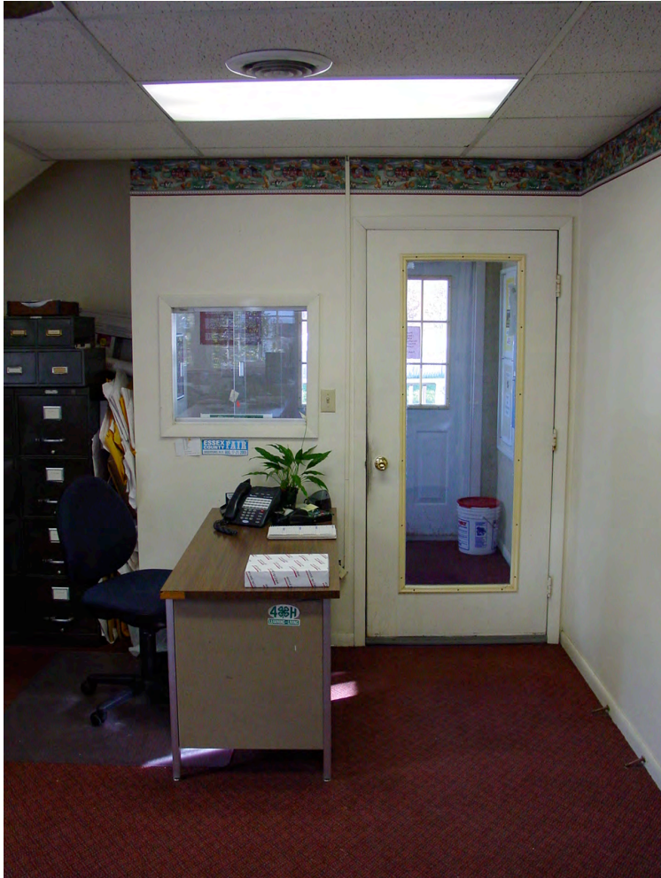
AI-5: Reception area with suspended ceiling, painted gypsum board wall finishes, and stair enclosure to second floor.
