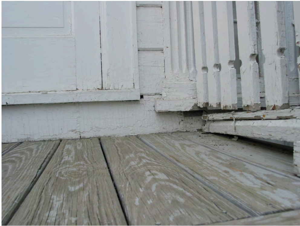
EC-5b: Railing deterioration at southeast entrance landing.
