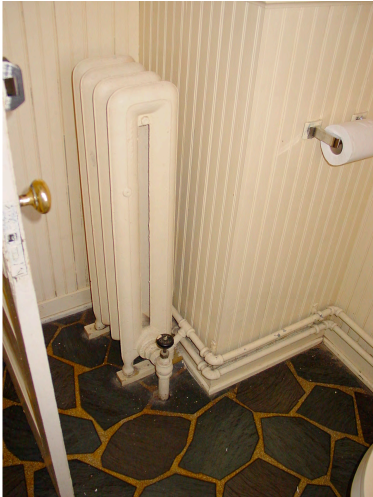
EC-5a: Single pipe radiator in second floor toilet room with exposed plumbing.
